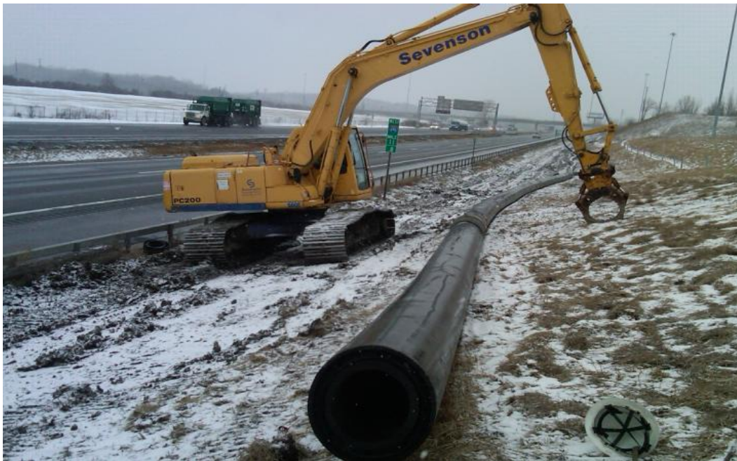
Slurry Pipeline Along 690
